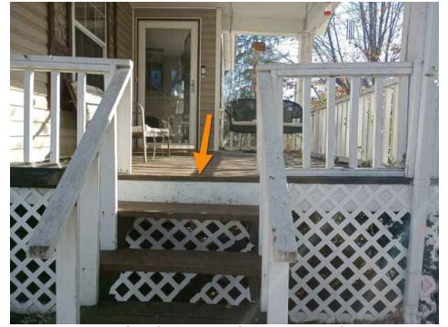
Front porch sloping downward
