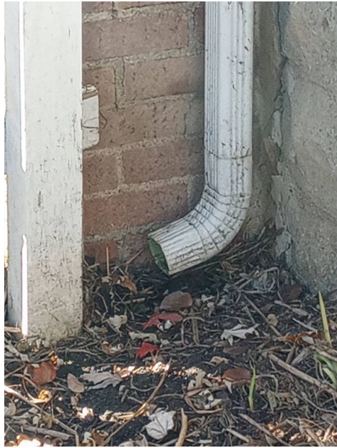
North side of chimney missing diverter tray
