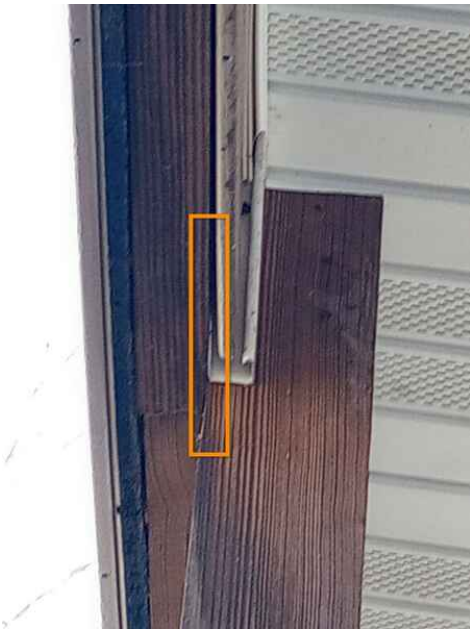
Not resting on the top of the post
