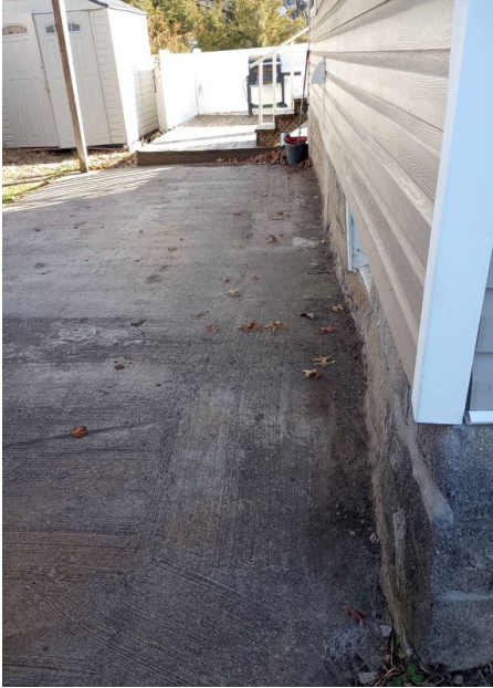
Concrete pad under carport is sloping towards the house
