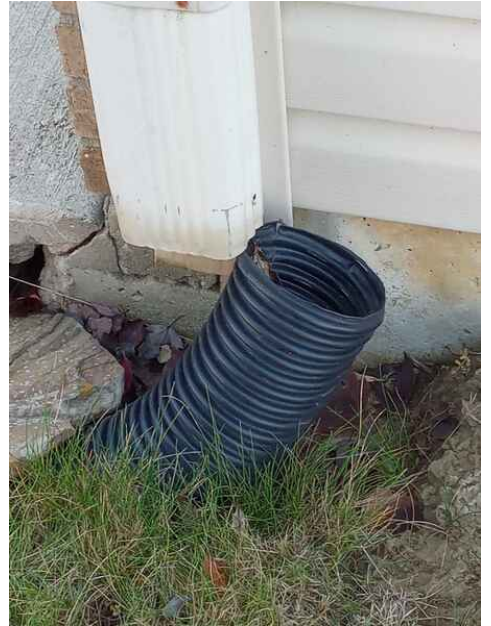
DETACHED PLASTIC PIPE-NEEDS TO BE REATTACHED
