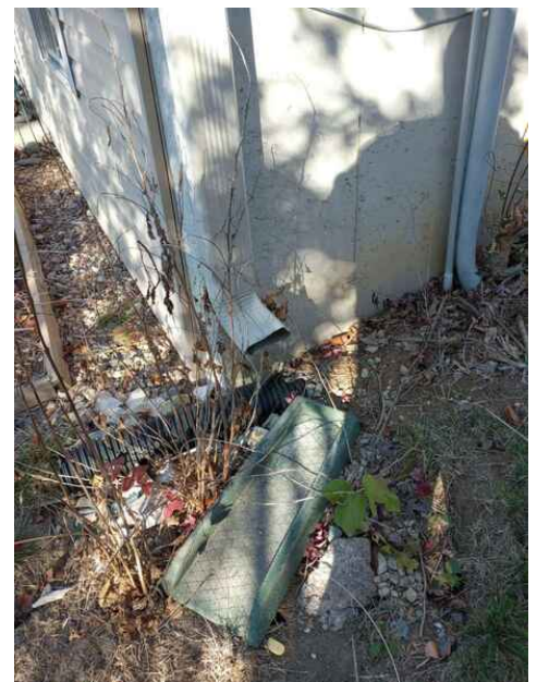
NEED INSTALL AN EXTENDER TO REACH THE SPLASH GAURD
