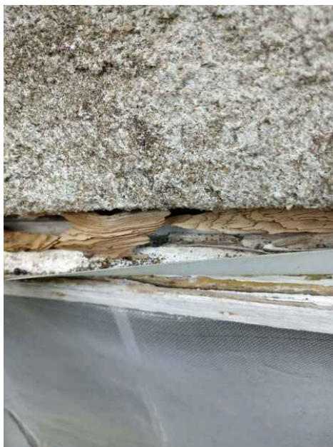
This is the window below the exit door. There is evidence of past ant damage. The damage is really old. No visible ants at the time of inspection
