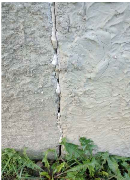
This crack on the basement wall should be resealed
