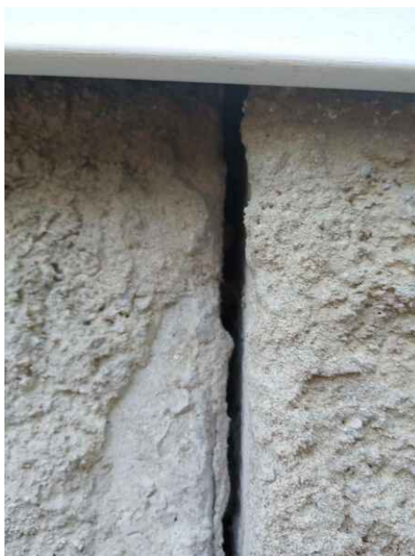
Crack to the right side of Garage door, should be sealed
